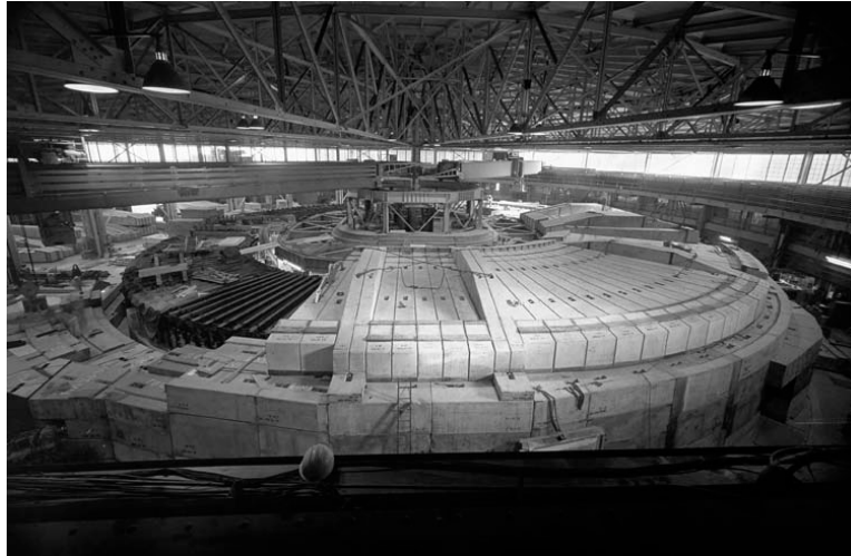
Figure 5. The installation of Moyer's roof shielding above the Bevatron in progress. The interlocking roof-blocks are keyed together with one another and to the supporting cylindrical shield wall so as to ensure seismic stability. Bending magnets of the synchrotron are clearly visible (1963). (Courtesy of Lawrence Berkeley National Laboratory)
